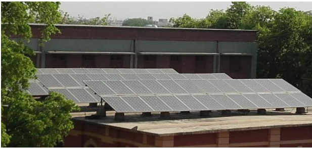
Fig.5. Normal Camera Photograph of Complete Solar Array
