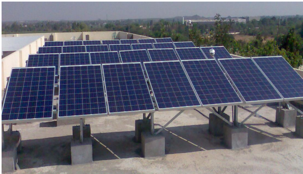
Fig. 2. Co-located ESS® multicrystalline and conventional poly-Si rooftop PV system at BVRIT
